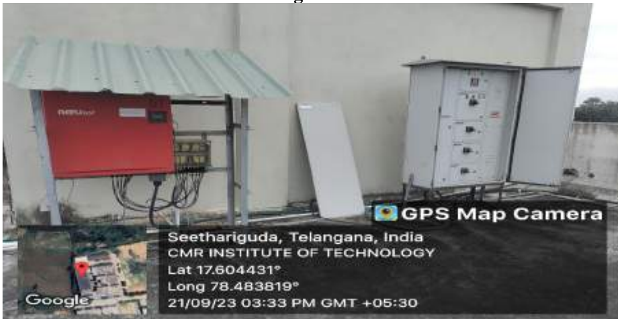
Inverter No : 1 & Grid Connection
