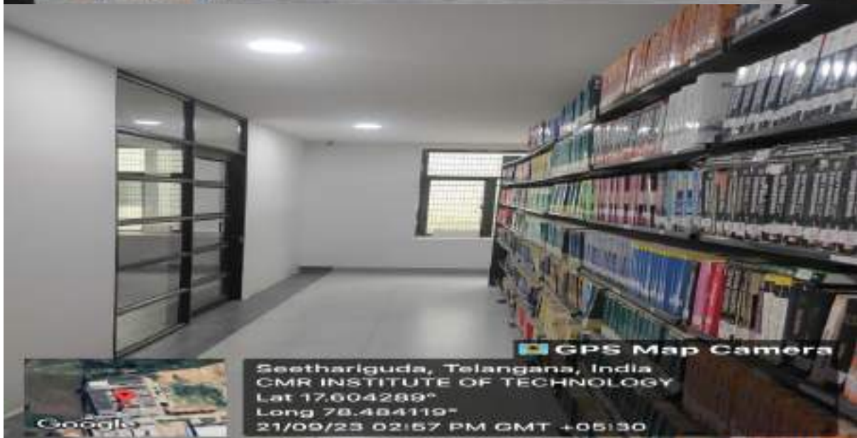
Led panels at Library
