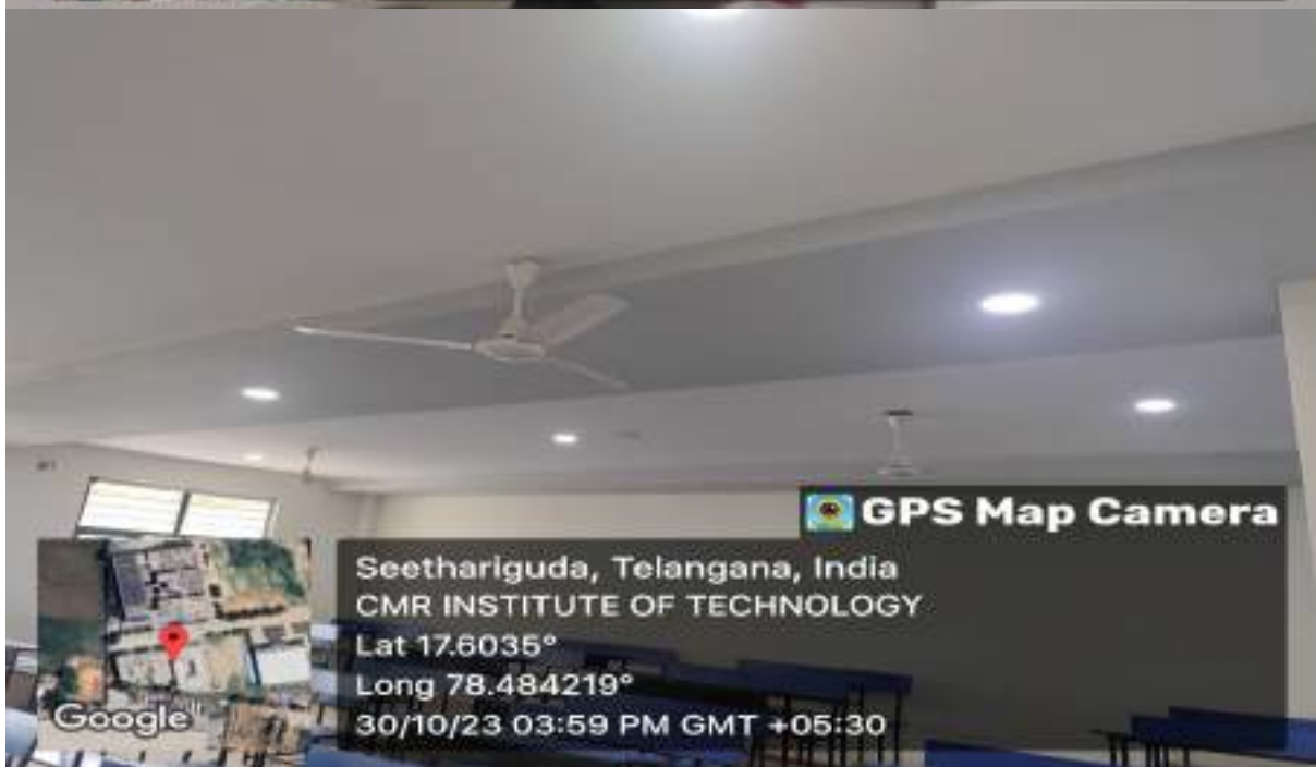
Led Panels at Class rooms & Labs
