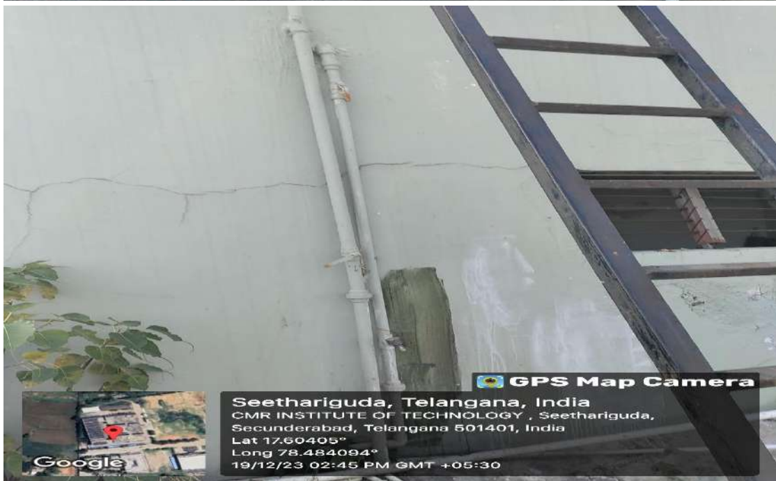
Distribution of Water from Tank
