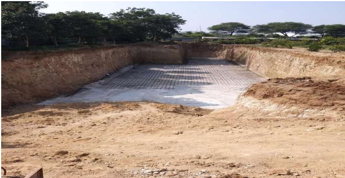
Sewage Water treatment plant
