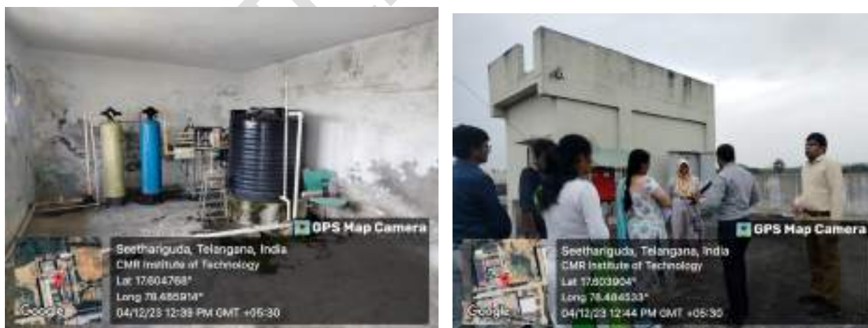
Plate 4: RO plant and rooftop water tank facility in the premises
