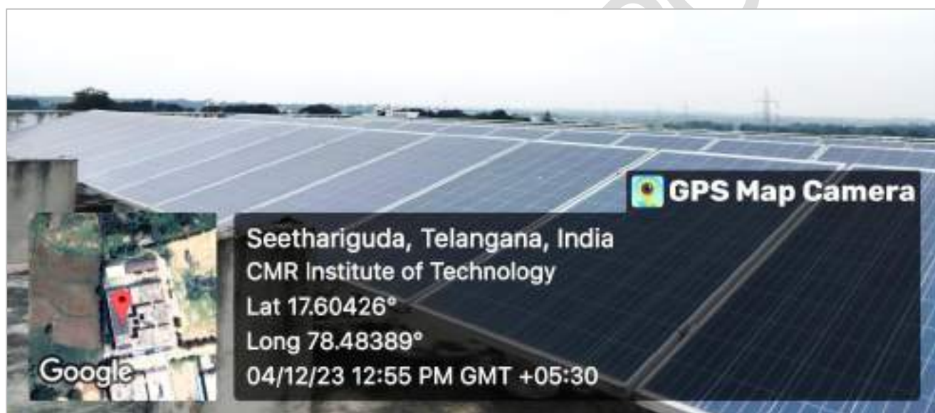
Plate 4: Rooftop solar panels in the campus
